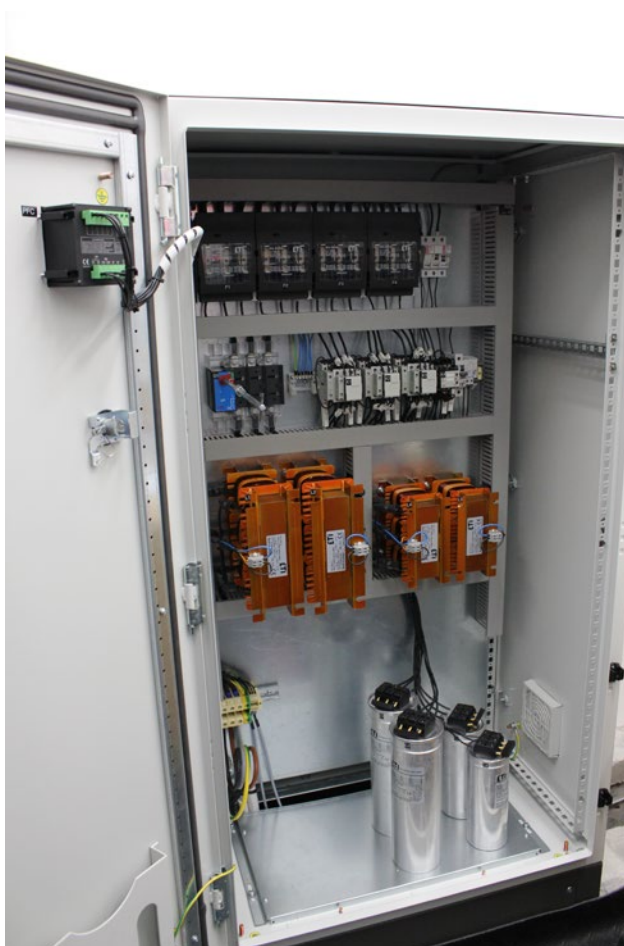
Automatic Power Factor Correction Banks
